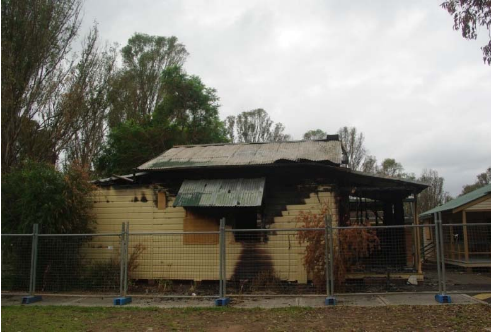
Plate A19 View toward western wall of the staff room, note extensive fire damage. (Source: RPS 2015)
