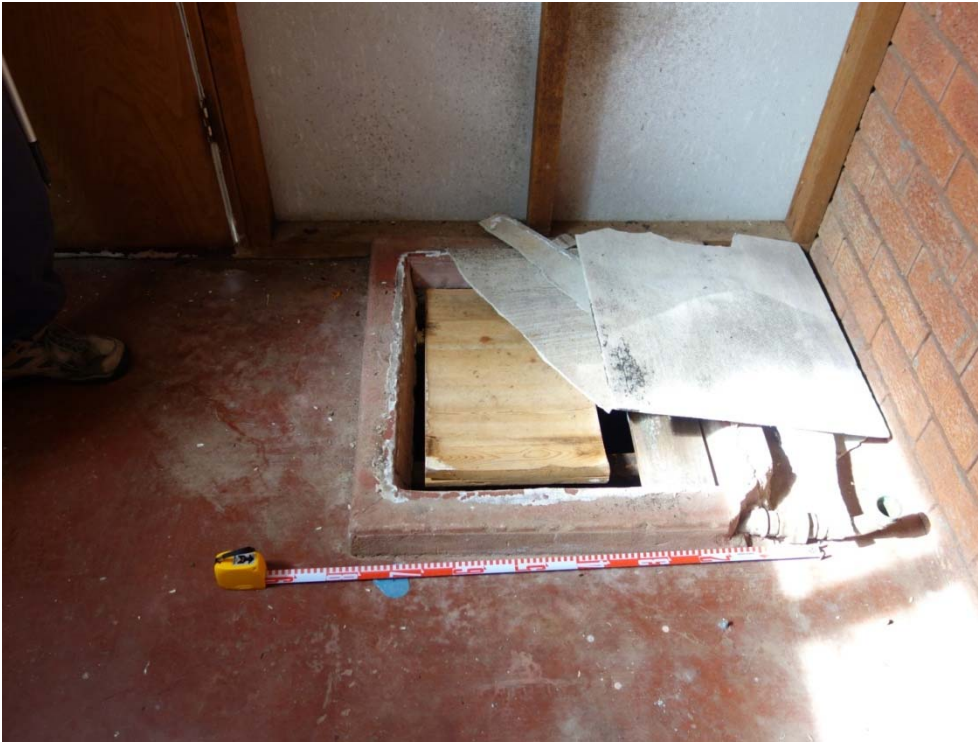
Plate A50 Internal sandstone lined well at 1972 The Northern Road, capped with fibro and timber. (Source: RPS 2015)
